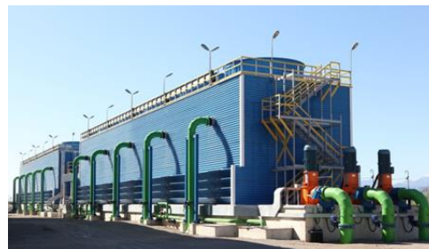
Figure 6. Cooling Tower Battery
