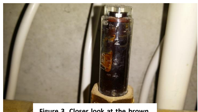
Figure 3. Closer look at the brown, slimy deposits caused by bacteria resulting in corrosion and fouling
