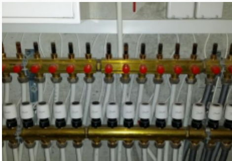
Figure 2. Heating system battery in an apartment building in Iceland
